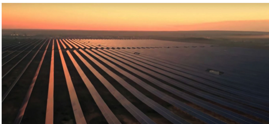
Solar panels, Neom project, Saudi Arabia, 2017 Excerpt from a promotional video available on discoverneom.com
