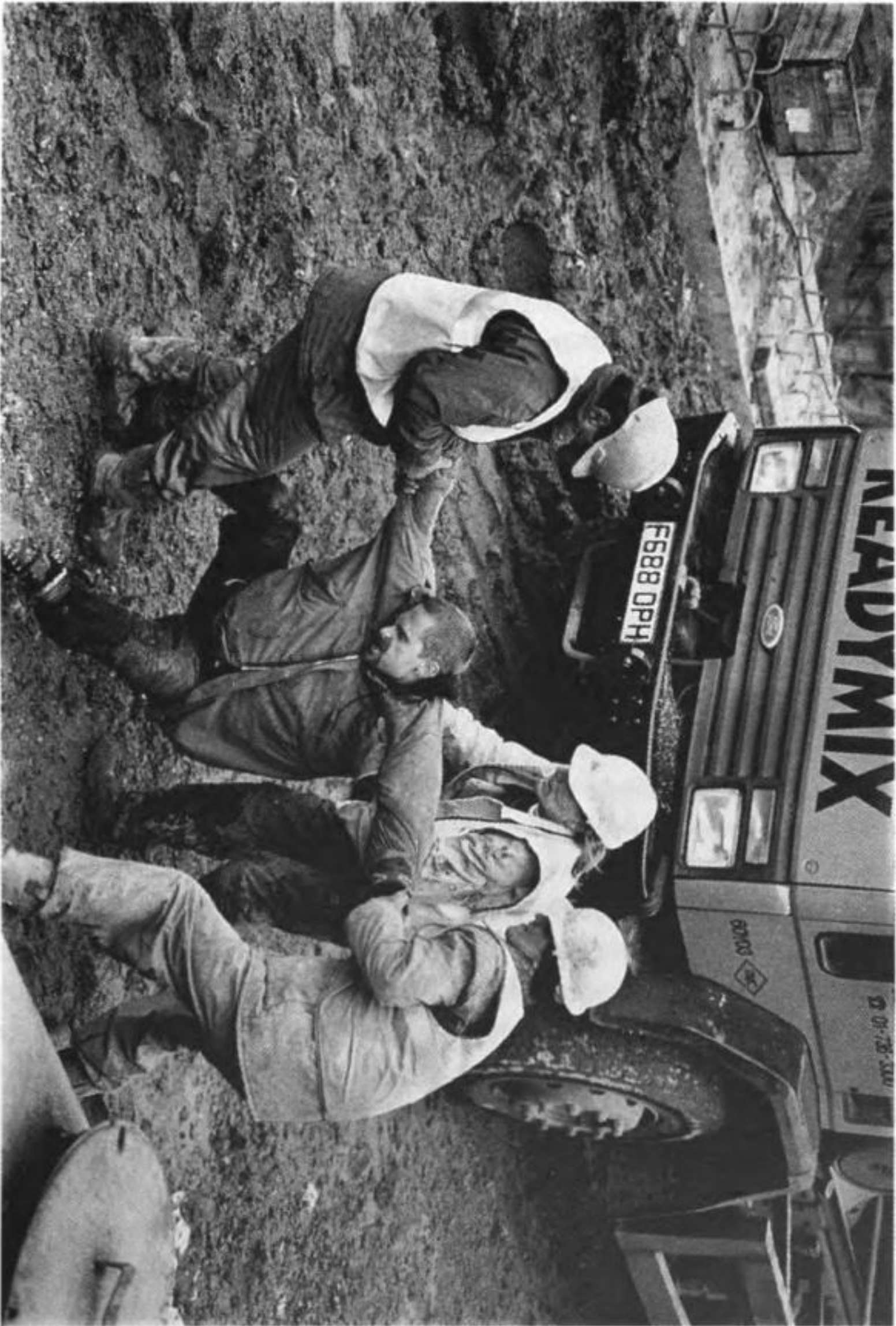
Worksite action on the M11 Link Road, early 1995. Photograph by Nick Cobbing
